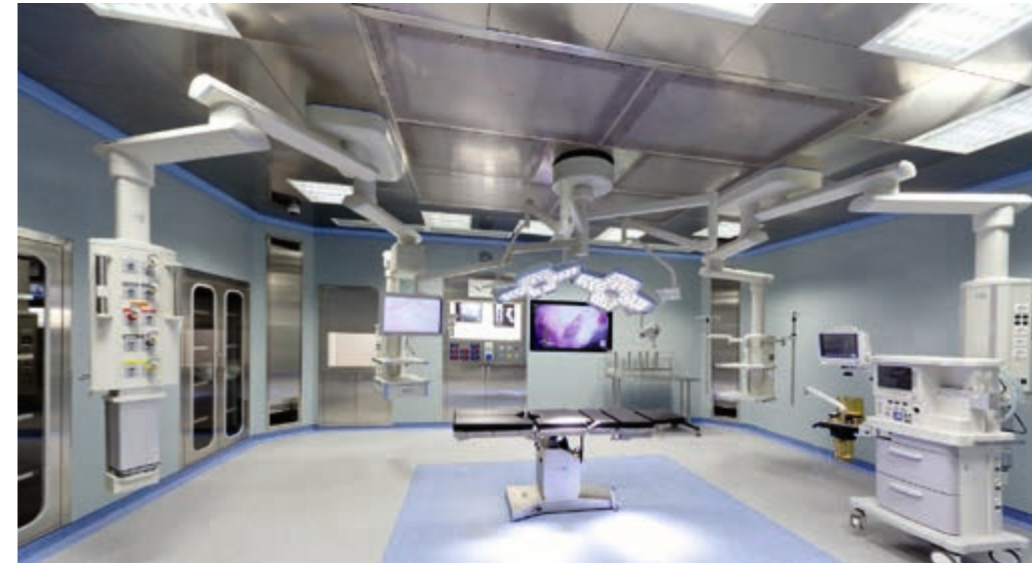
Operating Theatre At Casa Di Cura San Camillo Brescia, Italy | HIMACS aseptic prefabricated wall system: MED s.r.l. | Fabrication: 3MC s.r.l.
